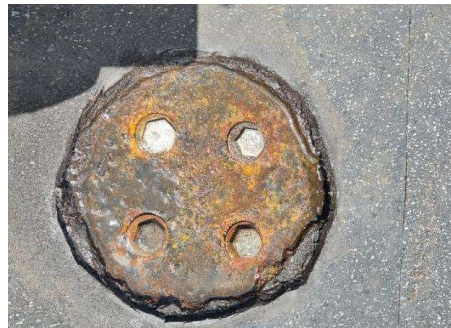
Failed Bolted/Welded Base Connection
